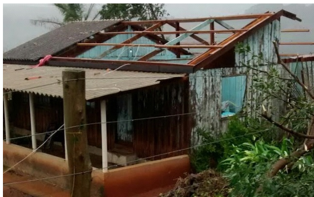
Figure 3: Photo of damage caused at home by alleged Tornado in Rosario do Ivaí [3].
