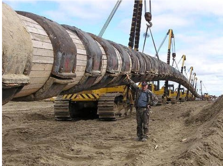
Building typical ground pipeline. Requires ground right of way and results in damage to ecology
